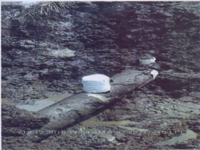
Figure 2: Wrapped cone on the pipeline.
